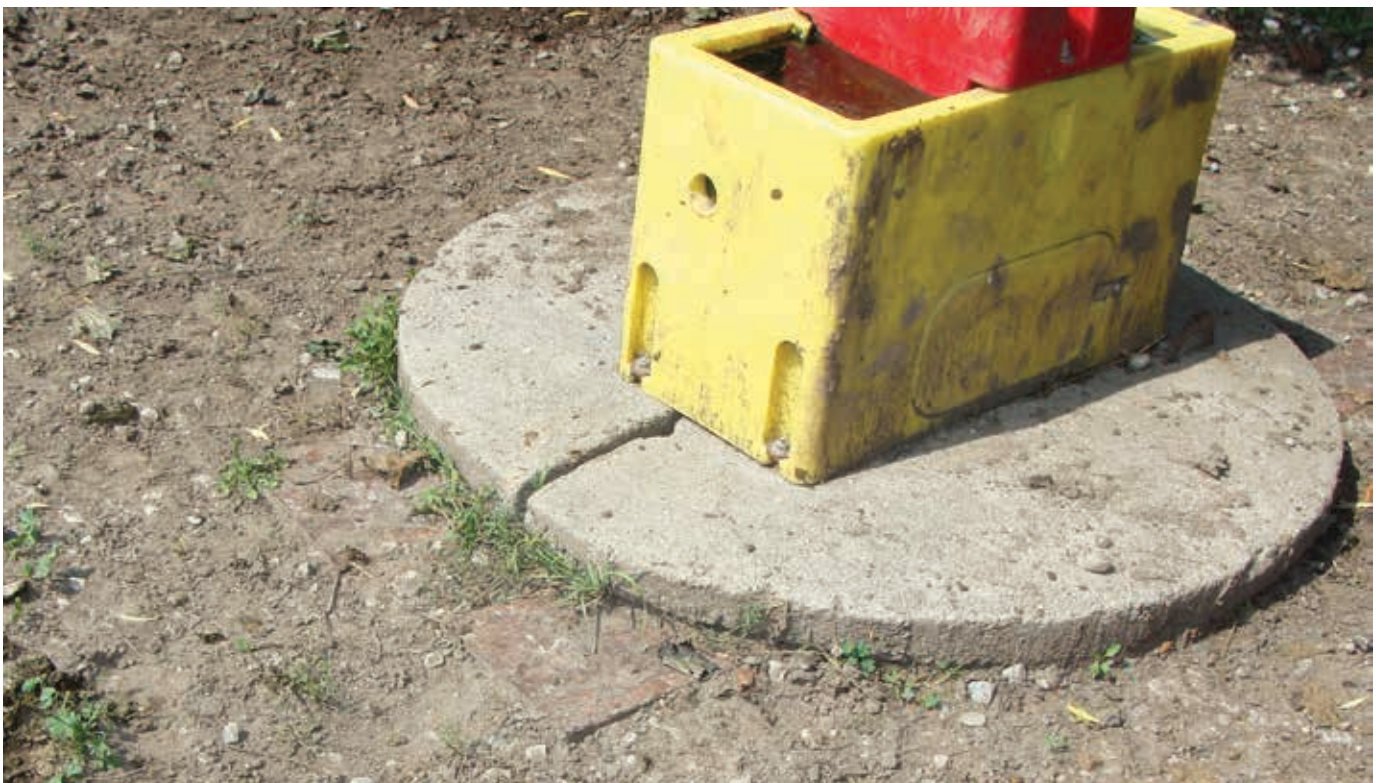
This picture shows the gap in the concrete well cap and its location in relation to the ground and potential sources of contamination.
