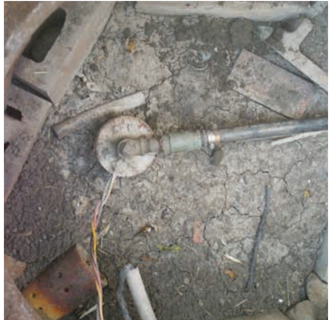
The soil is cracked, evidence that water has entered the well pit (not to be constructed this way anymore) and dried. One way to prevent this from happening is to upgrade the well by installing a pit-less adapter and extending the well casing at least 40 cm above the ground; and ensuring that construction/maintenance is conducted properly. New construction wells cannot be located in well pits. NEVER ENTER A PIT.
