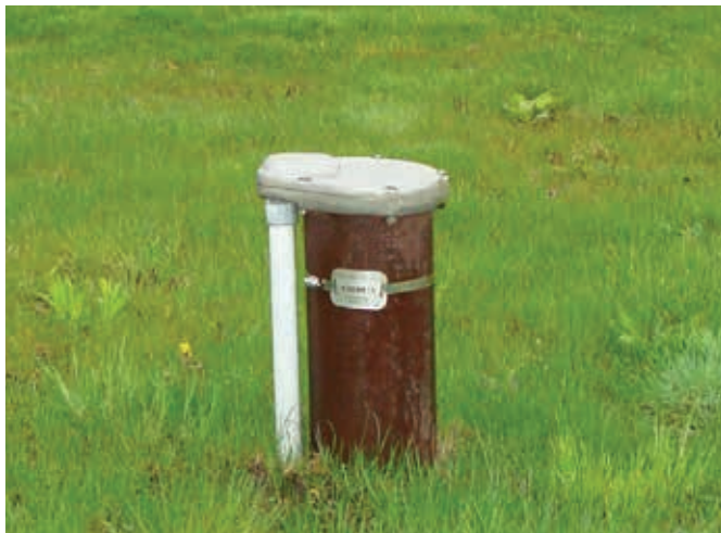
Properly constructed drilled well shown with a vented and vermin proof well cap, electrical conduit for submerged pump (to left of well casing), identification tag (linked to Water Well Record), casing extends at least 40 cm above the ground, and ground that is mounded away from well casing.
