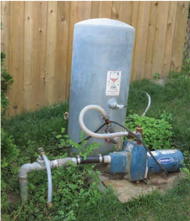
A well point (sand point) with a pump and pressure tank on the ground. These types of wells work in areas where the water table is high as they are not very deep. They are susceptible to surface contamination and changes in water table level. This well is used during the warmer months and winterized for colder months. Plumbing can also be installed below the frost line for year round use.
