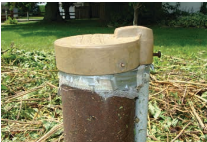
An inadequate well cap may allow pests and other types of contamination to enter into the well, and may not allow for proper ventilation.
