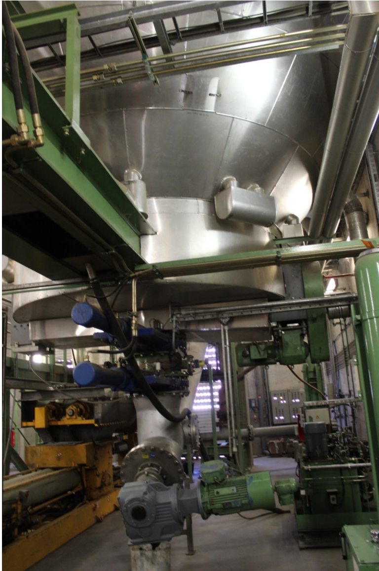
Figure 3-4-8 Anaergia, OREX, Kaiserslautern: Base of the Digester
