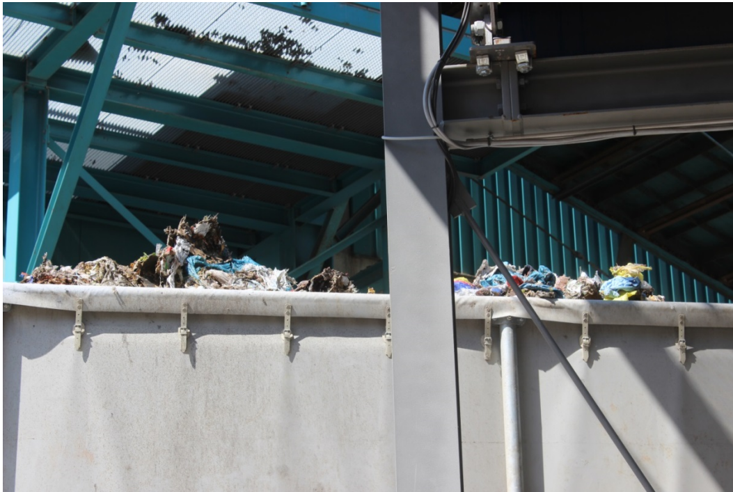
Figure3-4-6 Anaergia, OREX, Kaiserslautern: Dry Fraction Removed from OREX Press
