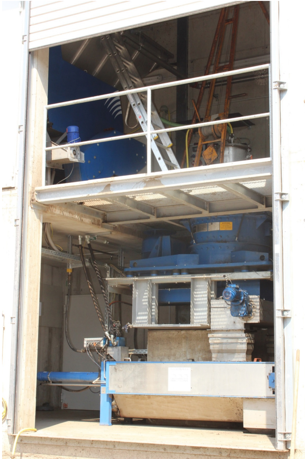
Figure 3-3-3 FITEC, Rothmuhle Biogas Plant: Biosqueeze Unit
