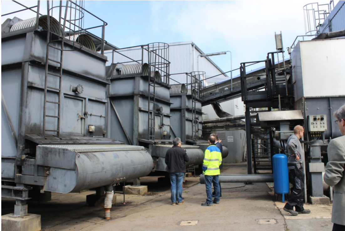
Figure 3-5-5 Veolia Passau: Horizontal Dry AD Units (3)
