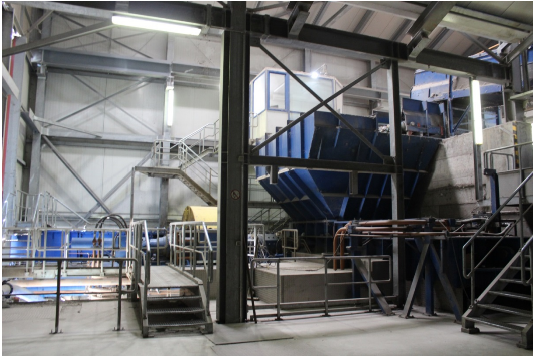
Figure3-4-4 Anaergia, OREX, Kaiserslautern: Feed Hopper (right), OREX Press (bottom left)
