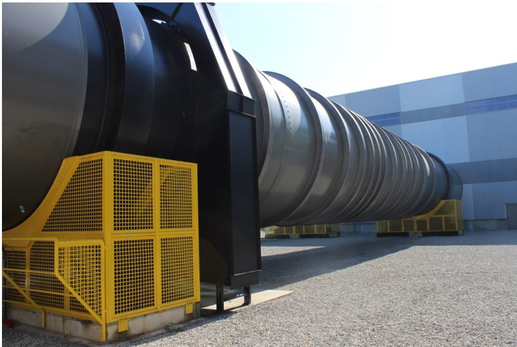
Figure 3-7-2 OWS Chagny AD Plant: Commuting Drum for MSW (start of process)
