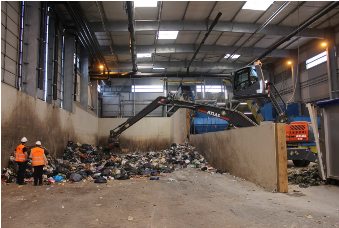
Figure 3-7-1 OWS Chagny AD Plant: Material Receipt and Loading Area
