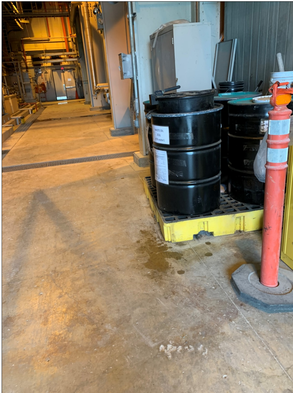
Figure 1: During the virtual site visit, a small quantity of liquid was noted on the floor beside the waste oil drum. The above picture was provided to BluMetric following the audit and was taken after the liquid had been wiped up.
