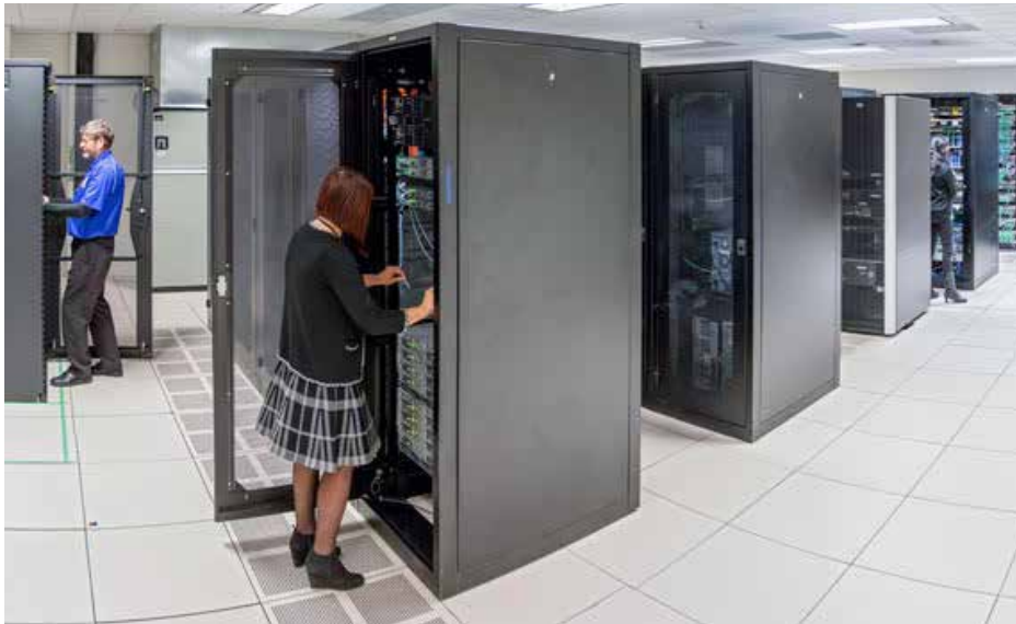
Figure 14: Regional server rooms. Cloud computing allows for data and applications to be centrally located and accessed by multiple devices
