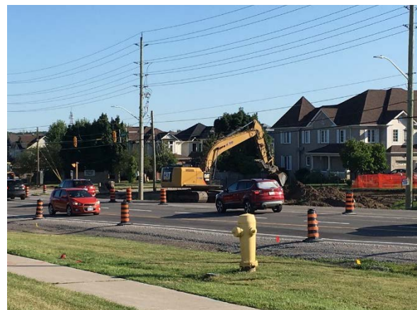
Figure 13: Brock Street widening construction, Whitby (Source: Region of Durham Planning and Economic Development Department)
