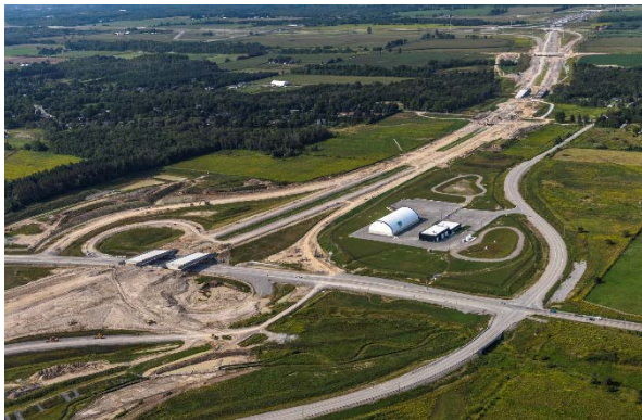
Figure 12: Highway 407, Phase 2 construction, looking southwest from the Bowmanville Avenue interchange (Source: Blackbird Infrastructure Group, August 2018)
