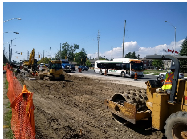
Figure 14: Highway 2 BRT construction east of Brock Road, Pickering (Source: Durham Region Works Department)
